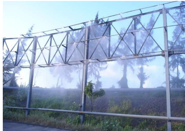
Dust Suppression System
