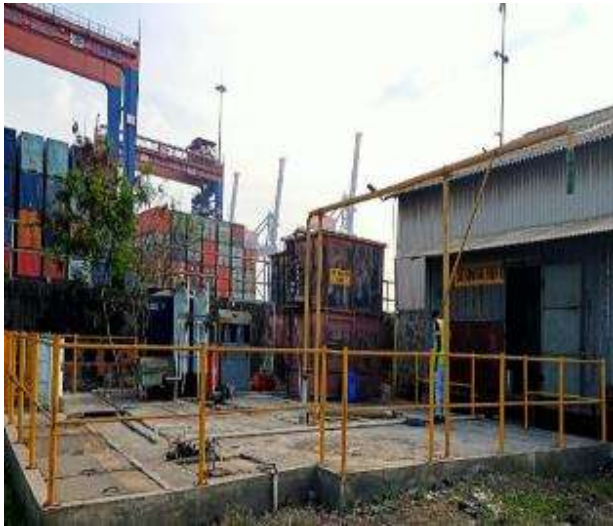
25 KLD STP at Port
